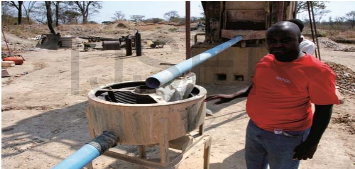
Figure 2.1: Picture showing gold processing plant.
